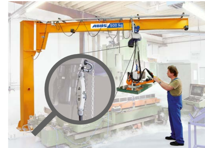
Jib crane with additional power socket and plug on hoist (Fig. 13)
